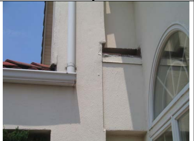
Photo 22. Difficult Scupper and Roof Detailing
