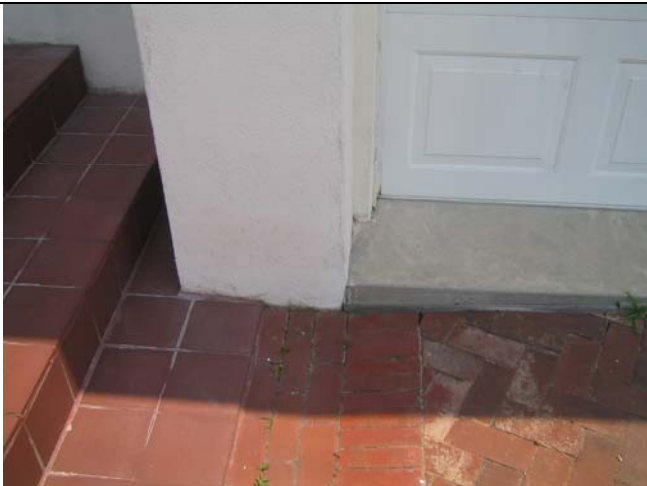
Photo 15. EIFS Below Grade
