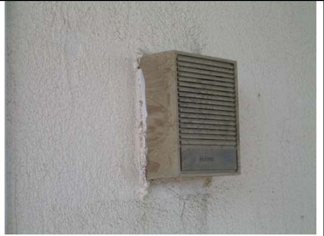
Photo 20. Poorly Sealed Fixtures
