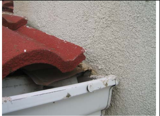
Photo 8. Missing Kickout Flashing
