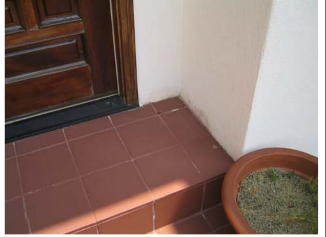
Photo 14. EIFS at Door and Stoop
