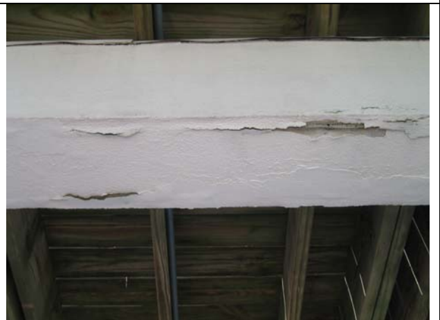
Photo 18. Moisture Damage to EIFS
